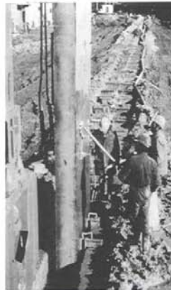
FIGURE 2.16 Workers apply a nonstick coating to a section of precast concrete slurry wall as it is lowered into the trench. (Courtesy of Soletanche)
